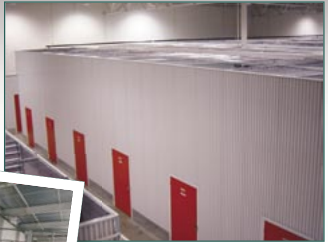
Island Mezzanine system shows external doors on first floor, and existing lighting systems.
